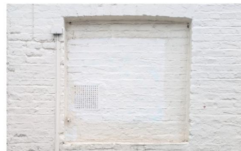
Front Elevation - Bricked in opening
