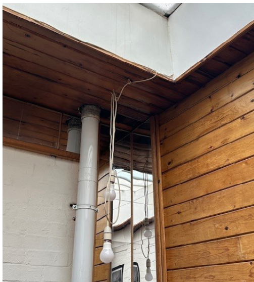
Exposed plumbing and electric wiring
