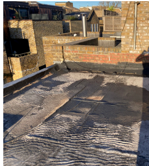
Roof is sagging and asphalt has failed
