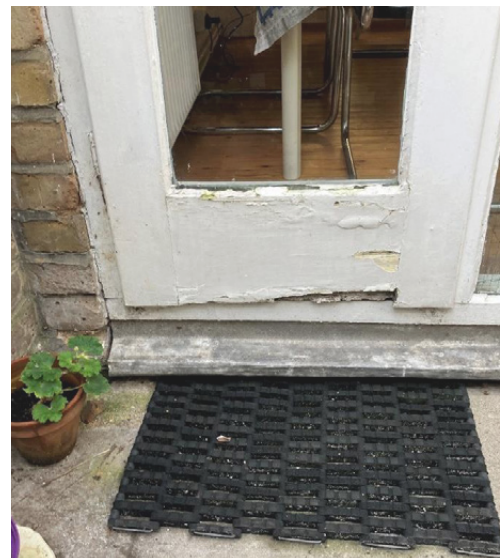
Advanced rot to timber doors and windows
