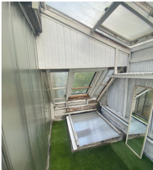
Rear infill construction is poor quality and leaking
