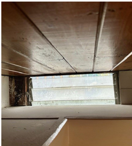
Single glazed louvre vents create draughts and heat loss
