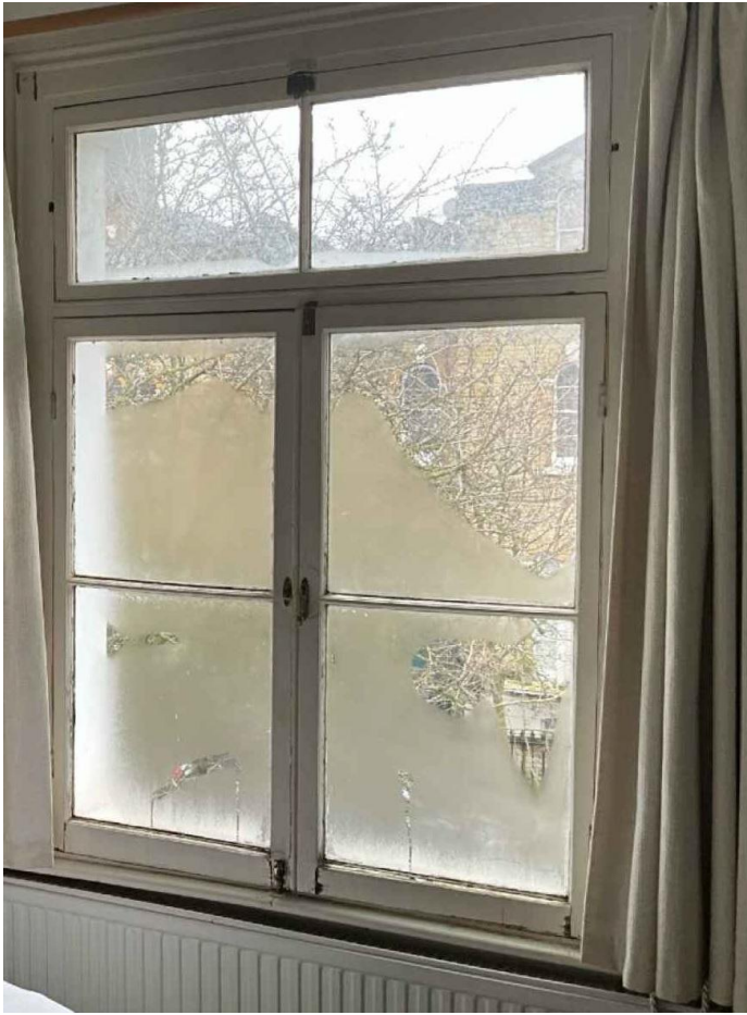
First front casement window that has been installed into a sash window frame
